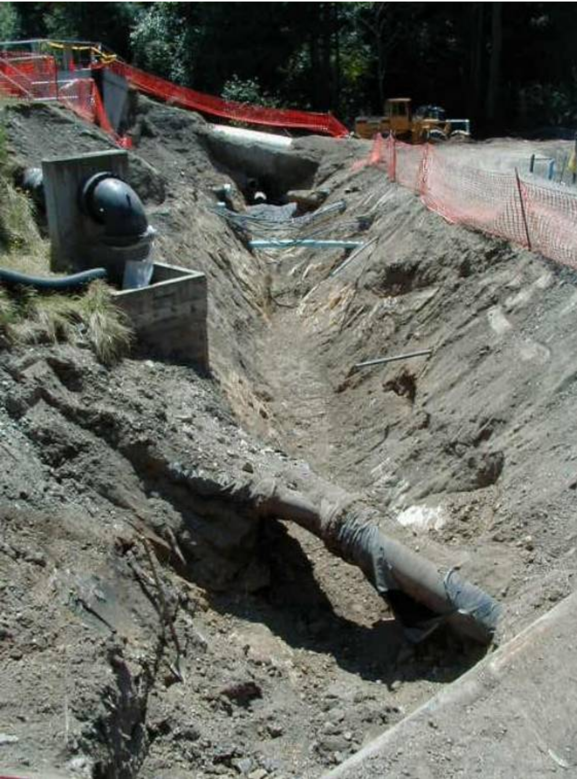
Photo 9-7. Photo of where the 277,200 gallon gasoline leak occurred (copyright 1999 nwcitizen.com. Reprinted with permission ).
